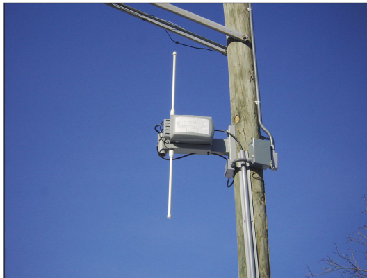
An outdoor Wi-Fi access point.
