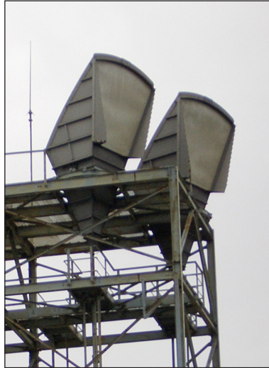
C-band horn-reflector antennas on the roof of a telephone switching.
