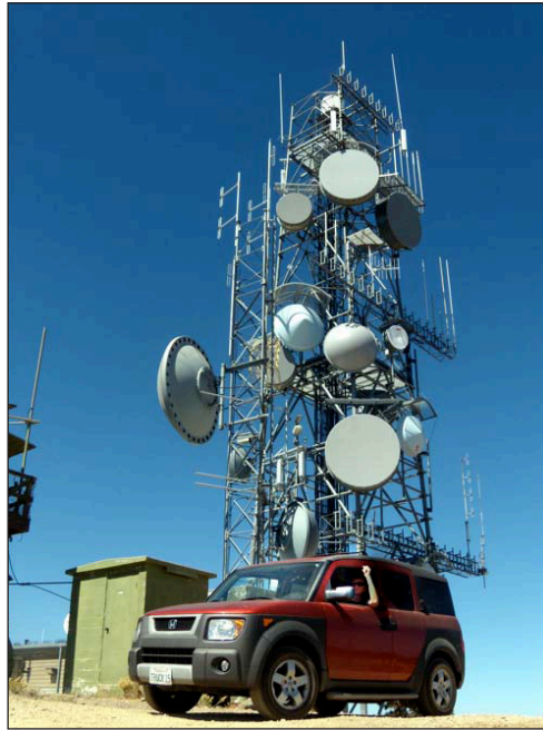
Communications tower with microwave relay dishes.
