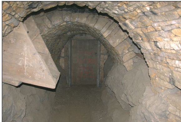
Door for directing ventilation in an old lead mine. The ore hopper at the front is not part of the ventilation.
