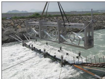
An example of helical-style Darrieus rotor turbines installed to capture energy from river currents, this technology is also employed for marine uses.
