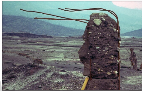
Building remnant in Francisco Leon destroyed by pyroclastic surges and flows during eruption of El Chichon volcano in Mexico 1982. Reinforcement rods in concrete bent in the direction of the flow.
