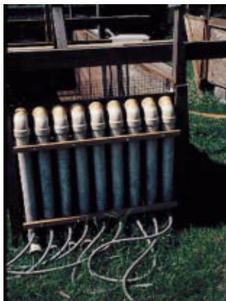
Figure: Air-lifts attached to a sheet of plywood at the front of raceway, showing garden hose attachment at a water depth of 32 inches
