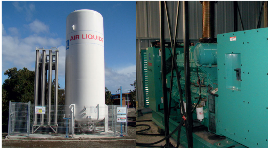
Figure: Oxygen tank and emergency electrical generator
