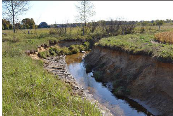
Bank erosion involves the undercutting and scouring of natural stream and drainage channel banks.
