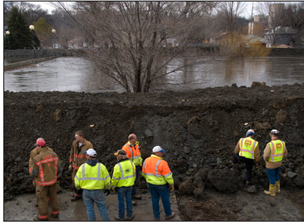
Slope instability issues for a temporary flood control levee in North Dakota.
