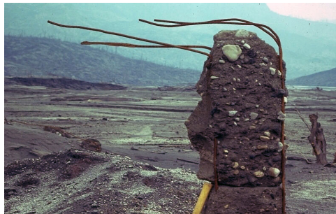
Building remnant in Francisco Leon destroyed by pyroclastic surges and flows during eruption of El Chichon volcano in Mexico 1982. Reinforcement rods in concrete bent in the direction of the flow.
