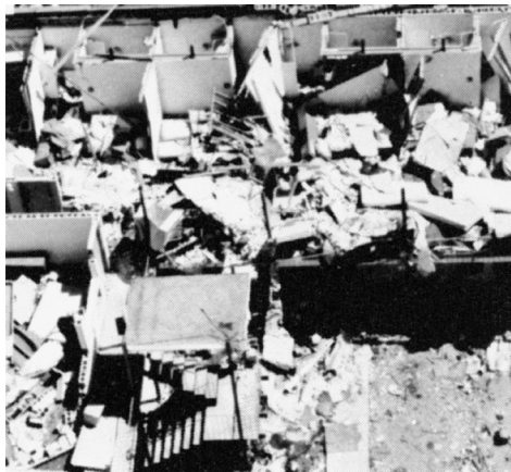
Multiunit building with its roof and many walls destroyed, the type of “severe damage” associated with strong tornadoes (ranking F3 on the Fujita Scale of tornado intensity).
