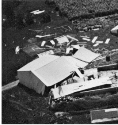
Machine shed pushed from its foundation, the type of “moderate damage” associated with weak tornadoes (ranking F1 on the Fujita Scale of tornado intensity).
