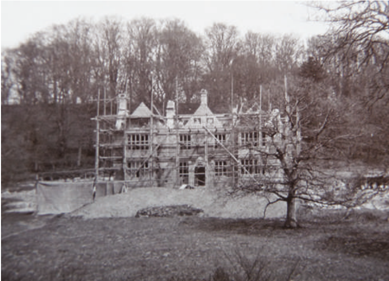
Fig. 18.4 Little Ridge under construction: the old Berwick St Leonard Manor House being rebuilt on its new site.
